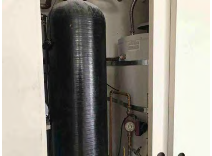
recirculating hot water and soft water tank
