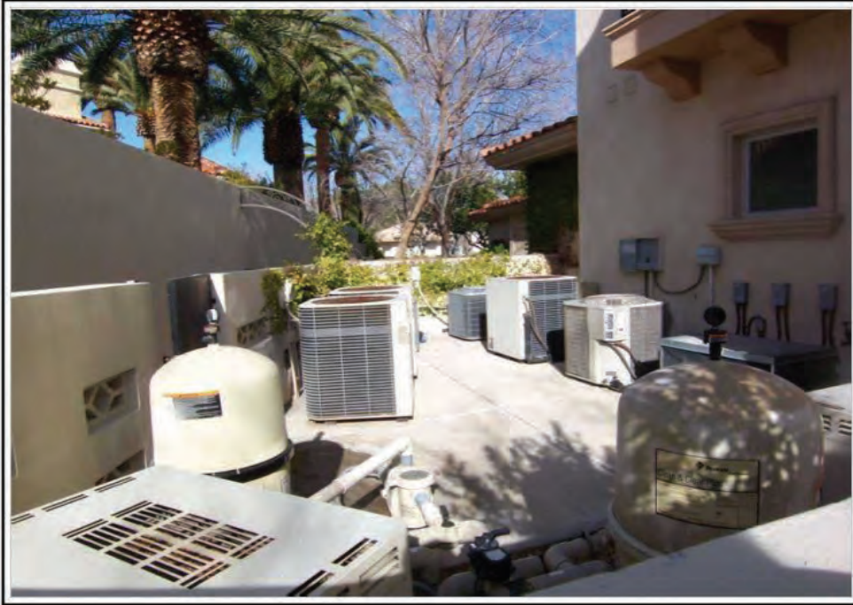
Side yard / Fenced mechanical area
