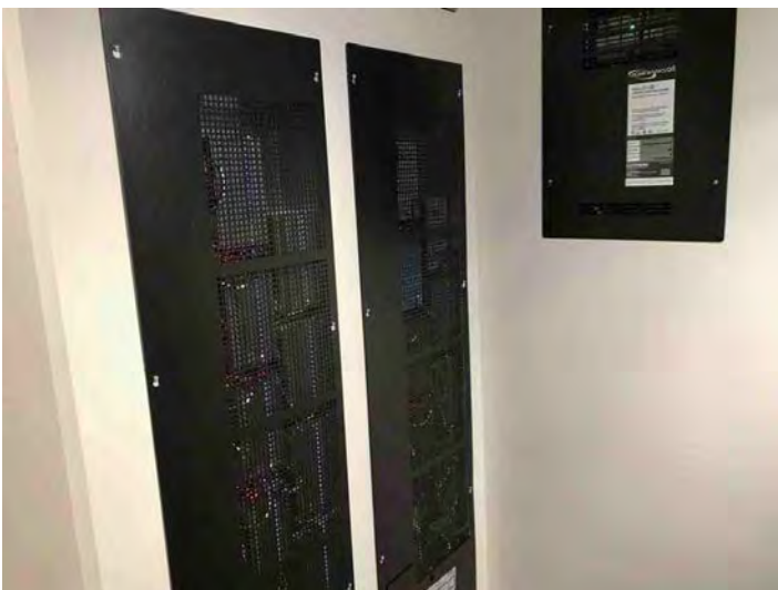
low voltage controller
